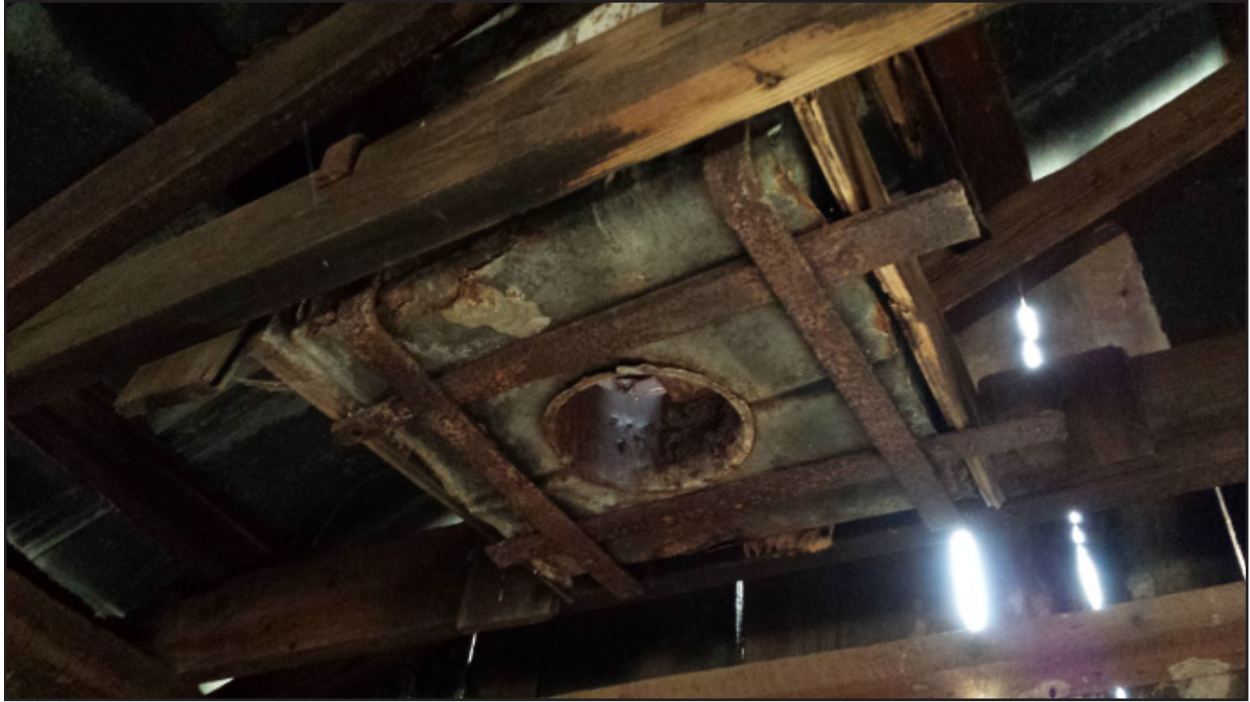
Figure 25. Wood stove chimney.
