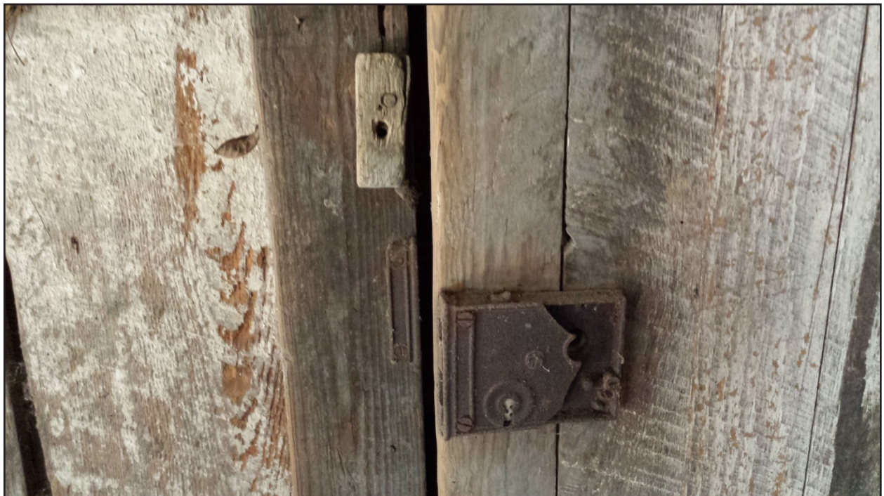
Figure 22. Metal lock and a wooden closure on the interior of a door.
