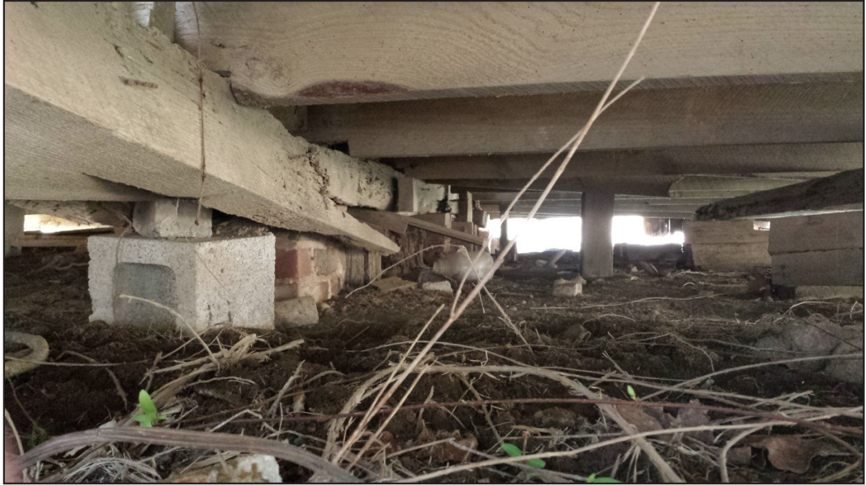
Figure 16. View of different types of piers used for foundation (cement blocks, bricks and mortar, and wood).
