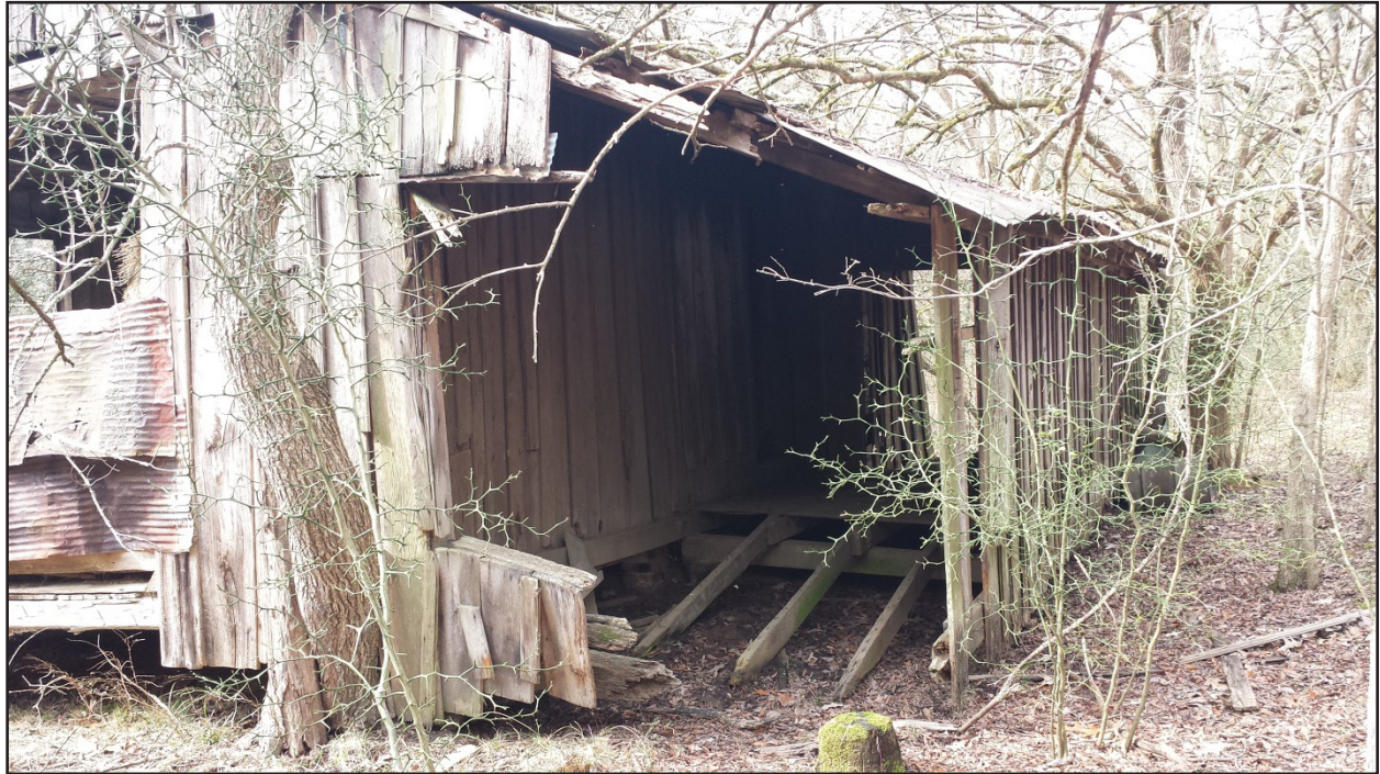
Figure 27. General view of the enclosed porch on the north side of SCH#9.
