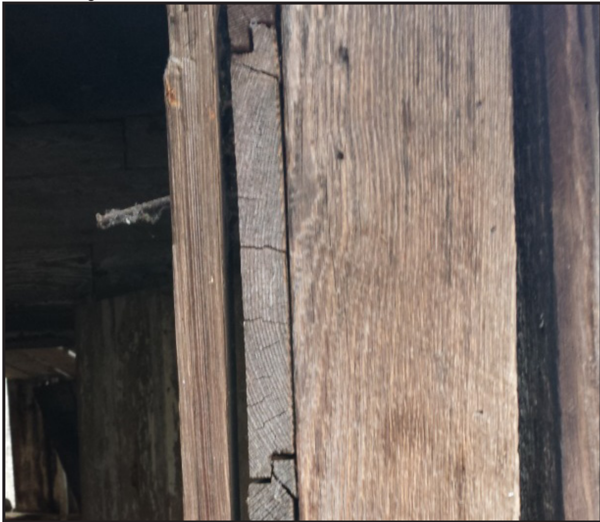
Figure 28. Boards with lap joints used in the construction of interior walls of a structure.
